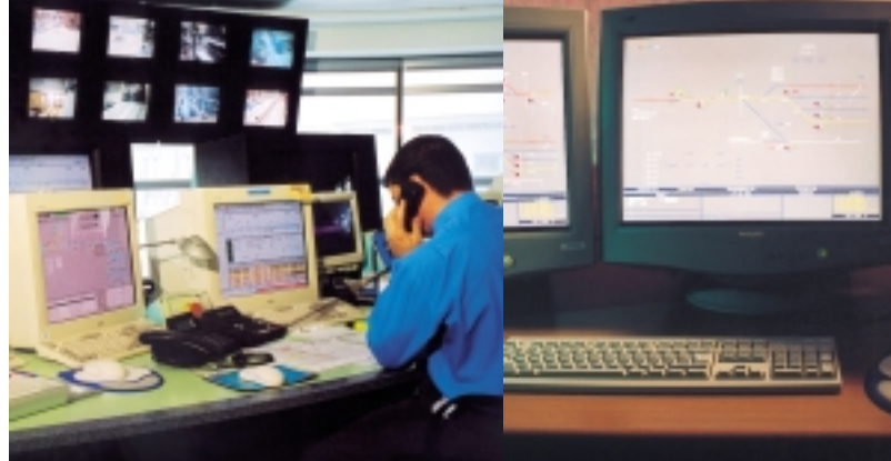
PRCI control station - Tramway
