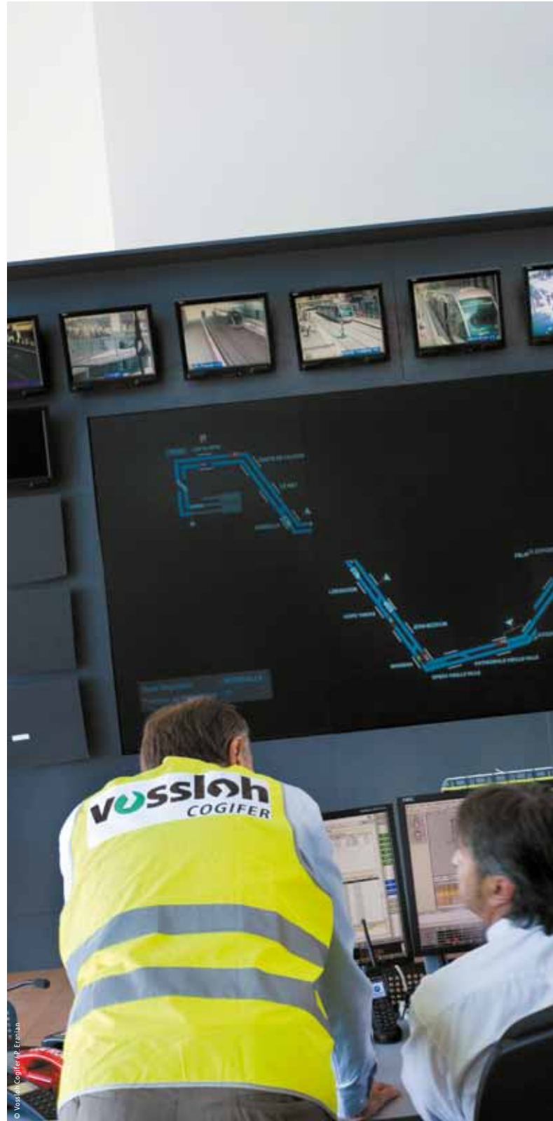
Tramway control station, Nice, France
